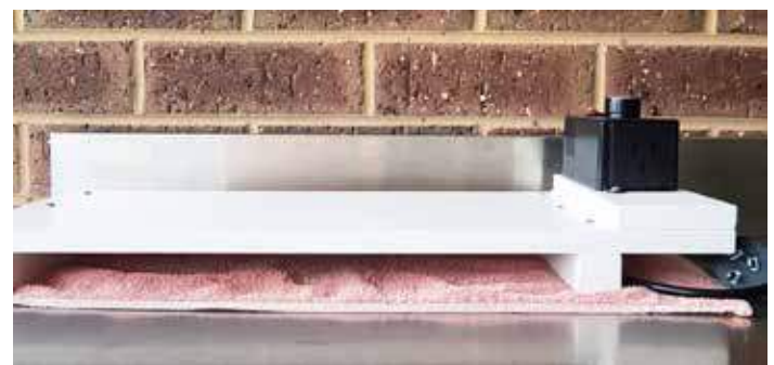
The new Regulator was mounted on a melamine shelving platform beside the machine.
